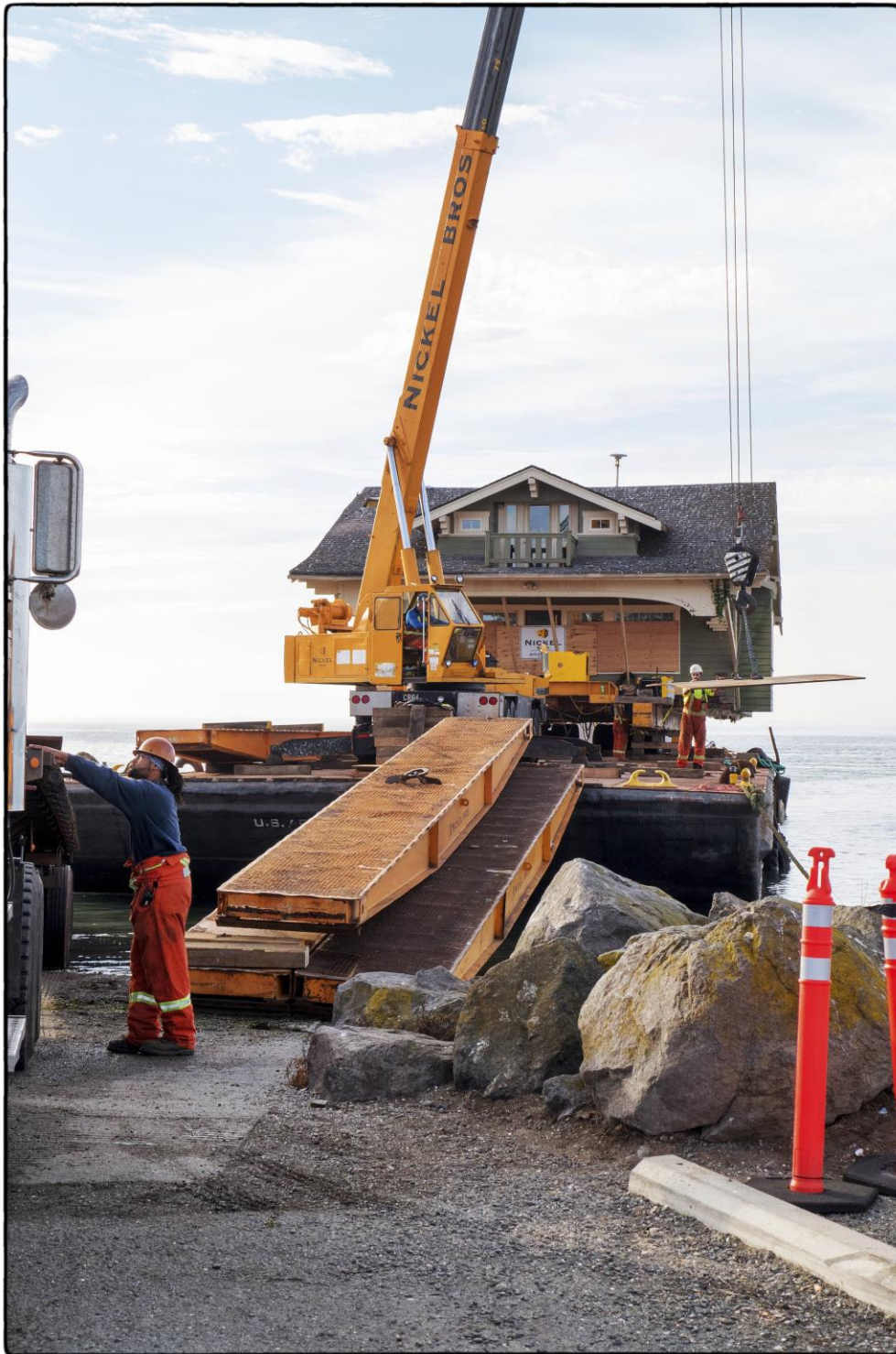
Crews from Nickel Bro. carefully unload Jim and Diane Luomas' craftsman home off a barge onto Cline Spit. Photo by Bob Lampert
